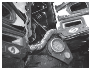
PermaDryPlus® intake gaskets installed dry: RTV used for end seals.
